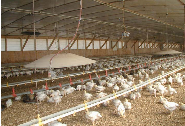
Illustration 4: A radiant heater used for brooding is shown above the feed and water lines
